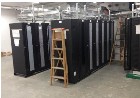
Racks in ARIEL room B1-08
