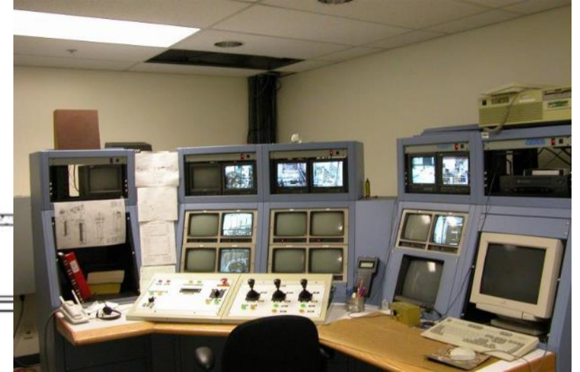
Remote crane control room
